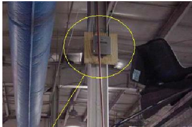
Figure 5-9 Access Point Mounted Directly to Steel Column
